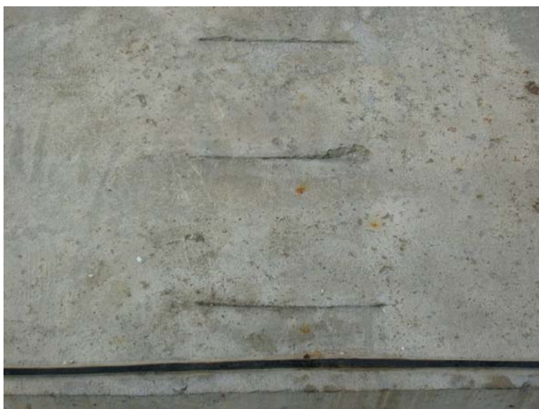
Figure 3.91 – Field test specimen ECR(DCI) (1) with simulated cracks at week 179, showing light staining on the surface.
