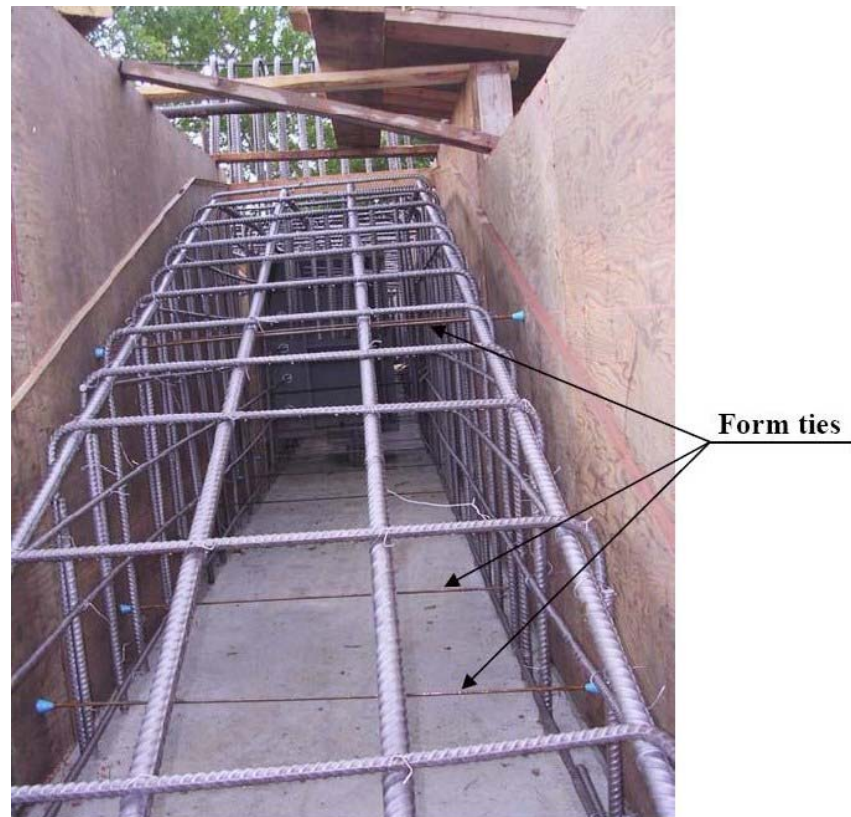
Figure 3.116 – Reinforcing bar cages at the east abutment for the Mission Creek Bridge, showing mild steel form ties used in the bridge decks.
