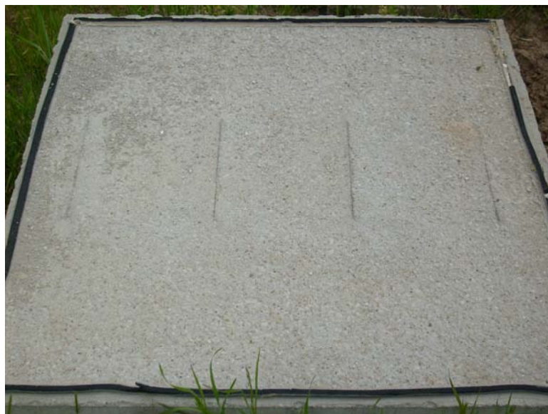
Figure 3.92 – Field test specimen ECR(Hycrete) (2) with simulated cracks at week 169, showing scaling on the surface.
