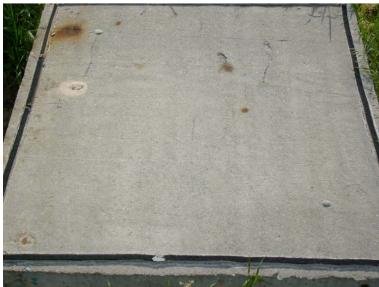
Figure 3.90 – Field test specimen Conv. (1) at week 205, showing cracking, spalling, and heavy staining on portions of the surface.
